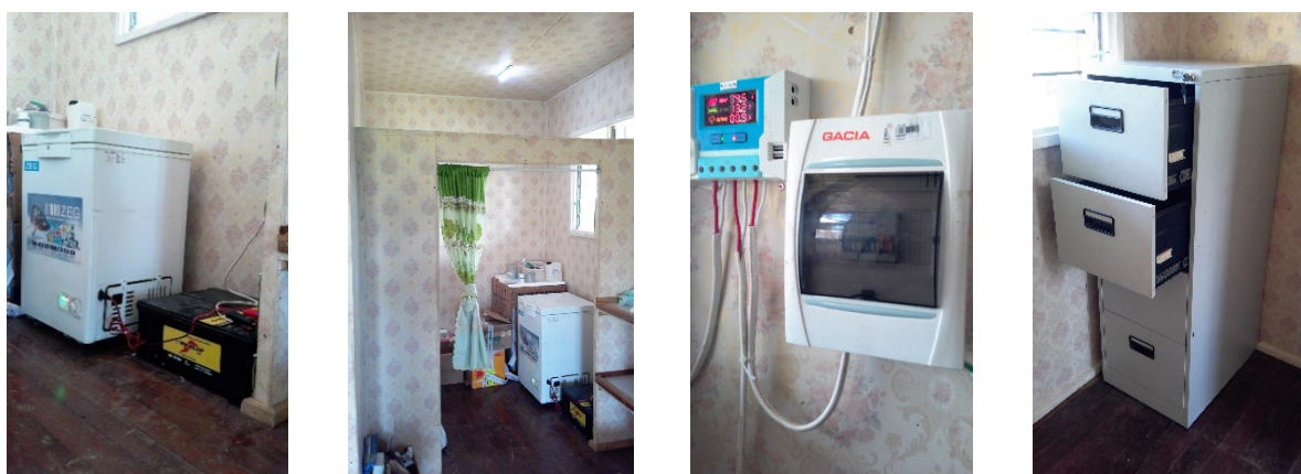
Figure 1: Fridge for the storage of medicines; storage area; solar power; filing cabinet for patient records
